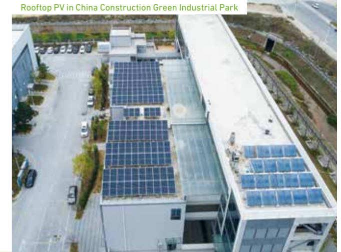
Rooftop PV in China Construction Green Industrial Park
